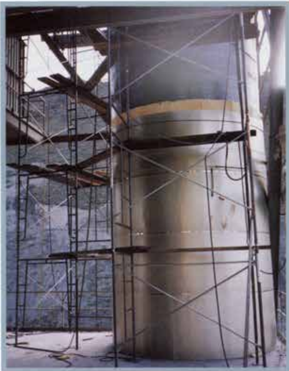
Field installation of insulation and cover on existing ductwork at an Eastern Oregon cement plant.
