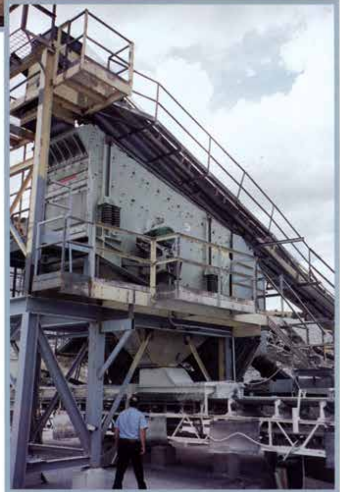
Field installation of a new screen and chutework on an existing cement plant in Eastern Oregon.
