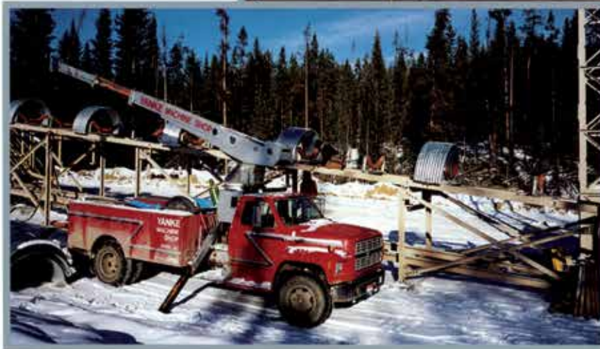
Field installation of a conveyor for a material handling system at an Idaho mine. ➤
