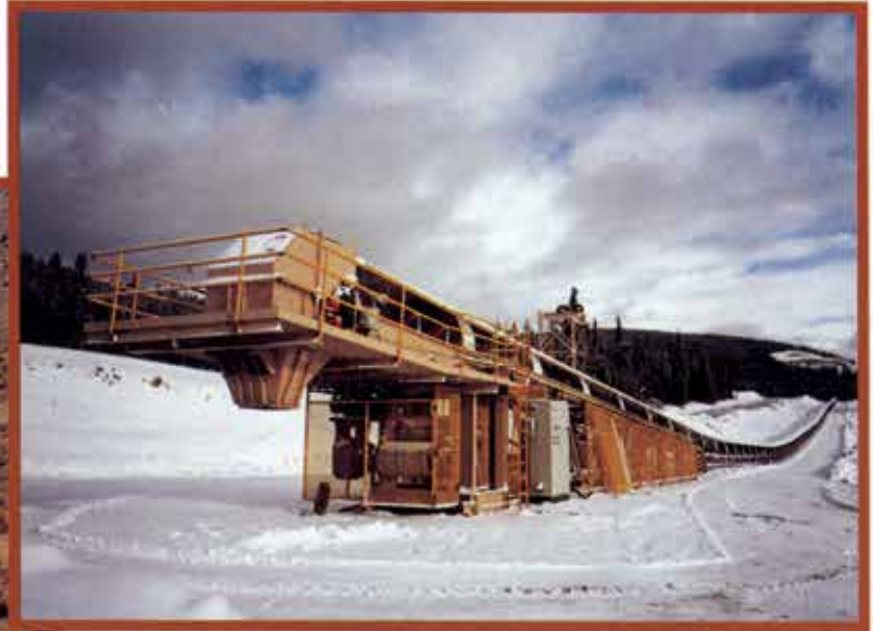
▲ Material handling conveyors, shop fabricated and field erected for a Central Idaho mining operation.
