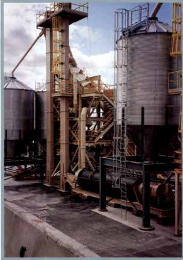
Field erection of structural steel and installation and assembly of piping and associated equipment for a perlite processing plant in Northern Nevada. ➤
